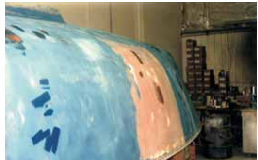
With new skin and core in place the repaired hull was faired before barrier coating and painting.
